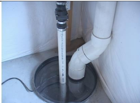
Pump Discharge and radon vent pipe.
