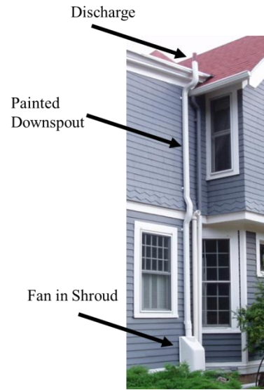
Fan located in shroud Downspout on exhaust painted to match trim colors
