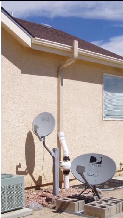
System located near other mechanical components
