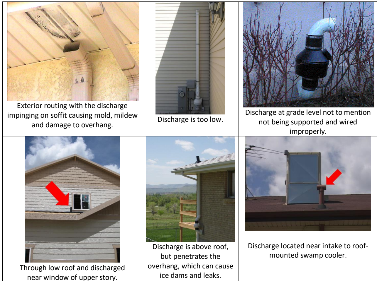
Figure 67: Improper Discharge Points
