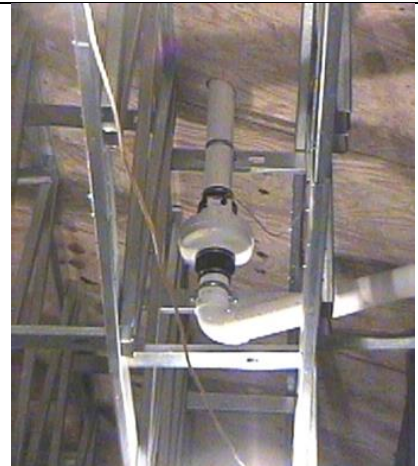
Concealed in attic when installed during construction
