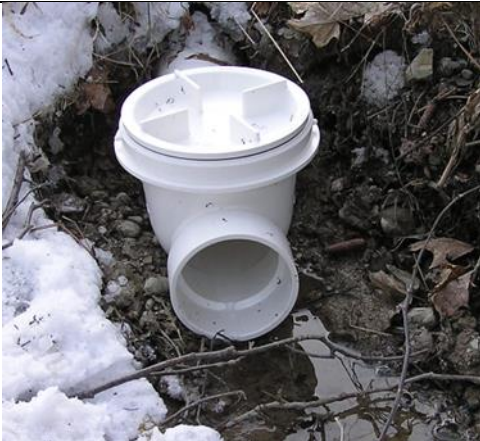
Soakaways on gravity drained systems to be fitted with full throat check valve. Referred to as Backwater Valves.
